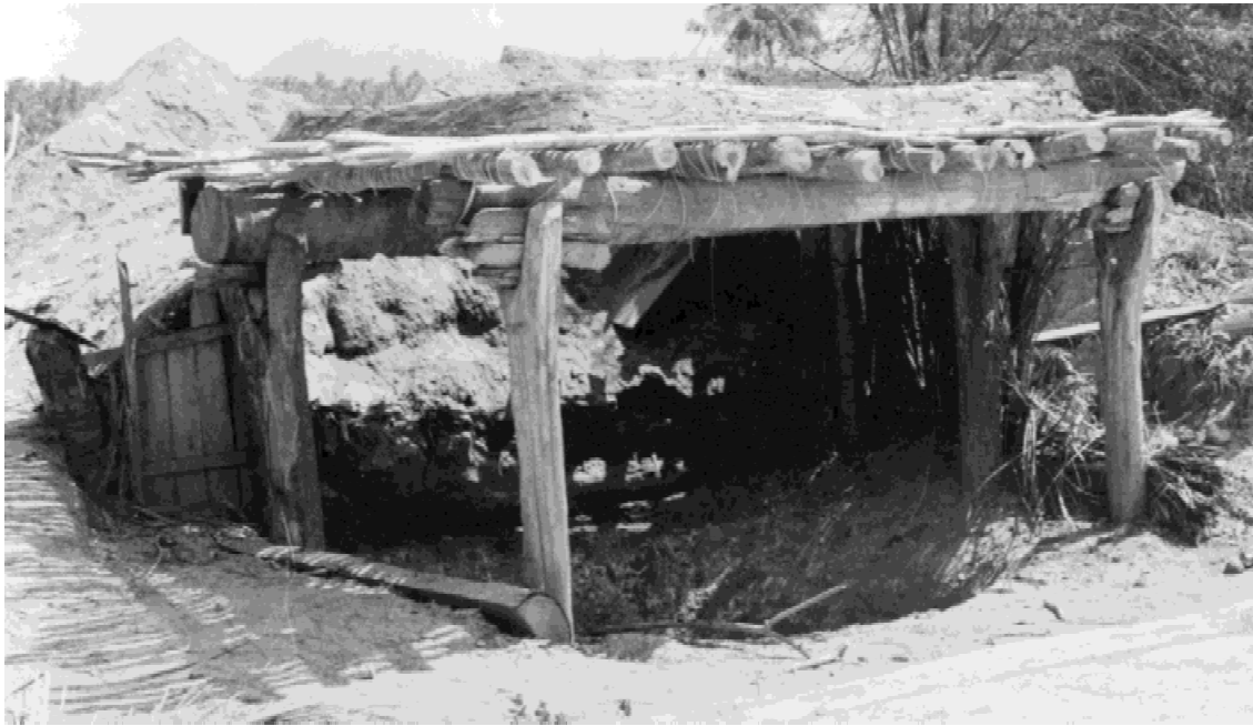
Figure 2. Filtering device, known as tapeixtle , used for leaching estuary water to produce brine. This tapeixtle is still under construction; the taza , or tank for storing brine, under the upper platform has yet to be coated with lime plaster.
