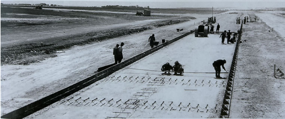
Figure 3. The construction of the reinforced concrete runway at Yeşilköy Airport, with its transverse and longitudinal steel supports, general view, c.1950. Sarıgöl, op. cit., p. 103 (used with permission).
