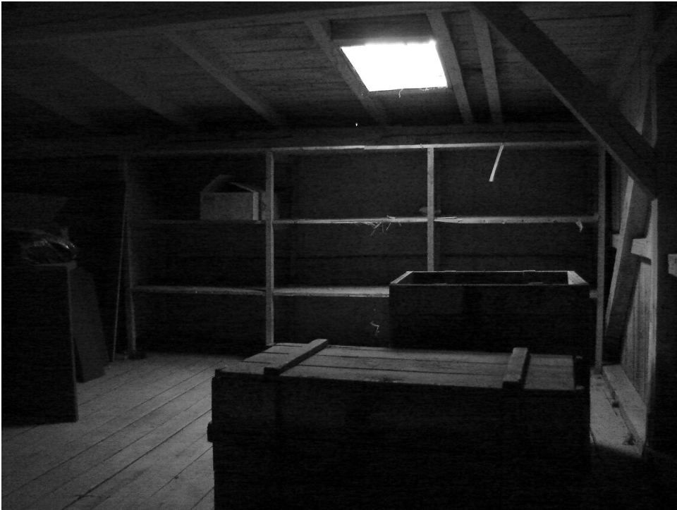
Figure 4. The attic of the old building of the Francisc I. Rainer Institute of Anthropology after a final clearing. Photographer: Alexandra Ion.
