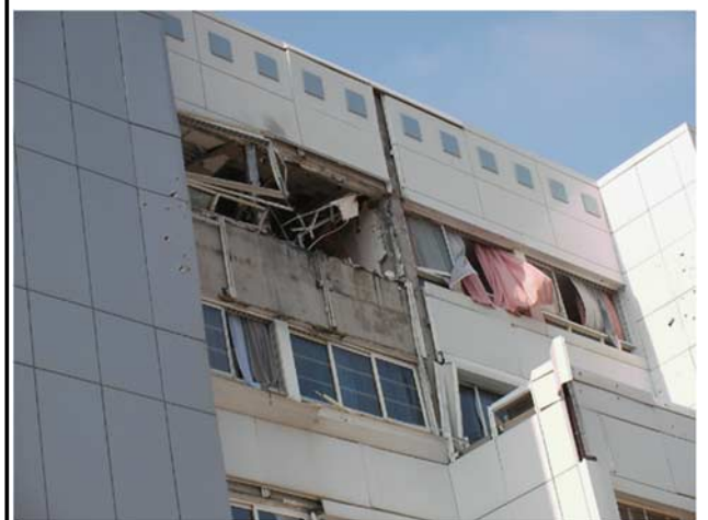
Damage Sustained by Western Galilee Hospital During the 2006 Second Lebanon War.
