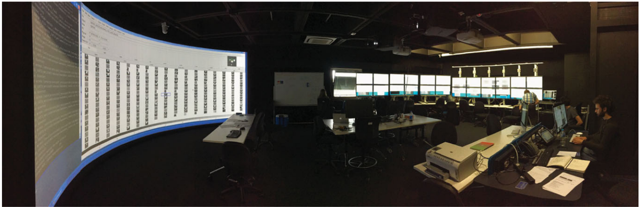
Figure 2. A panoramic view of the updated workspace for O2, showing the reconfigured TDW at the right of the image, the review, and control stations in the middle and the curved projection screen to the left.
