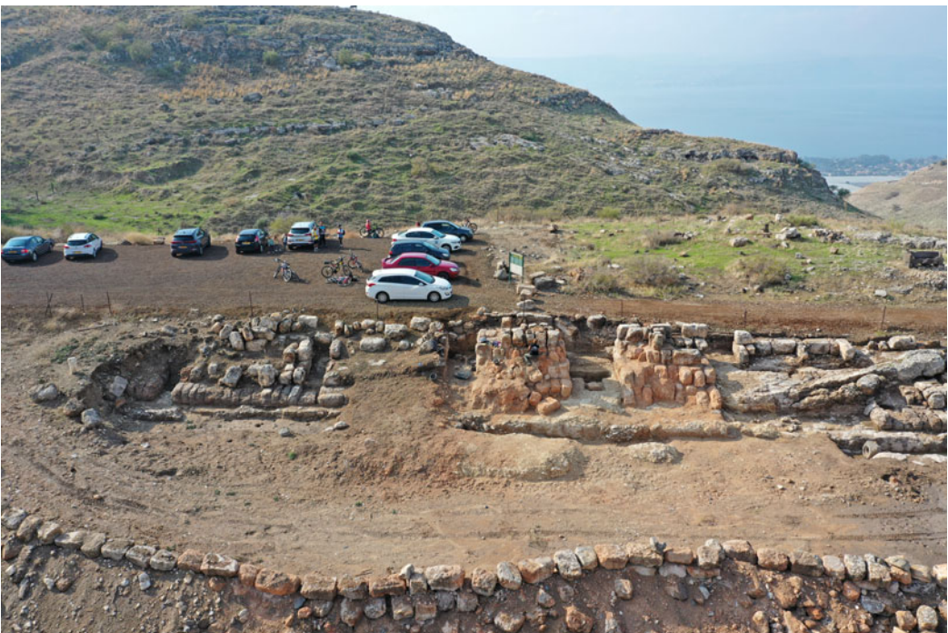
Fig. 12. The southern funerary podia (TT7–12) during conservation work, looking west. (M. Eisenberg.)
