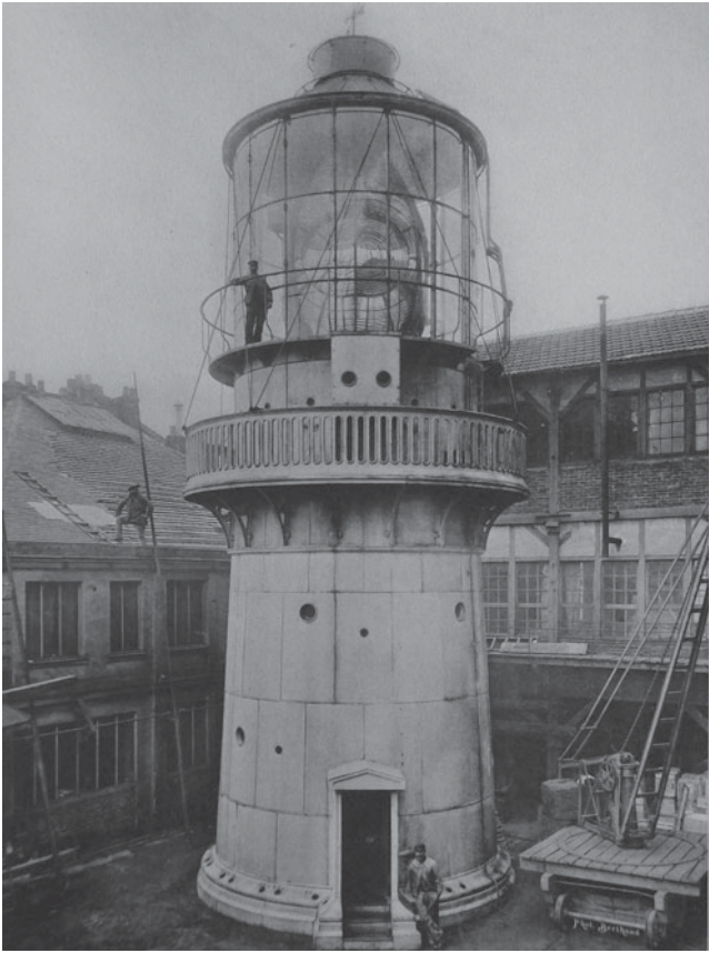
Fig. 2. Peiyüshan Lighthouse, under construction at Barbier Bénard and Turenne yard, Paris, c. 1894/5.
