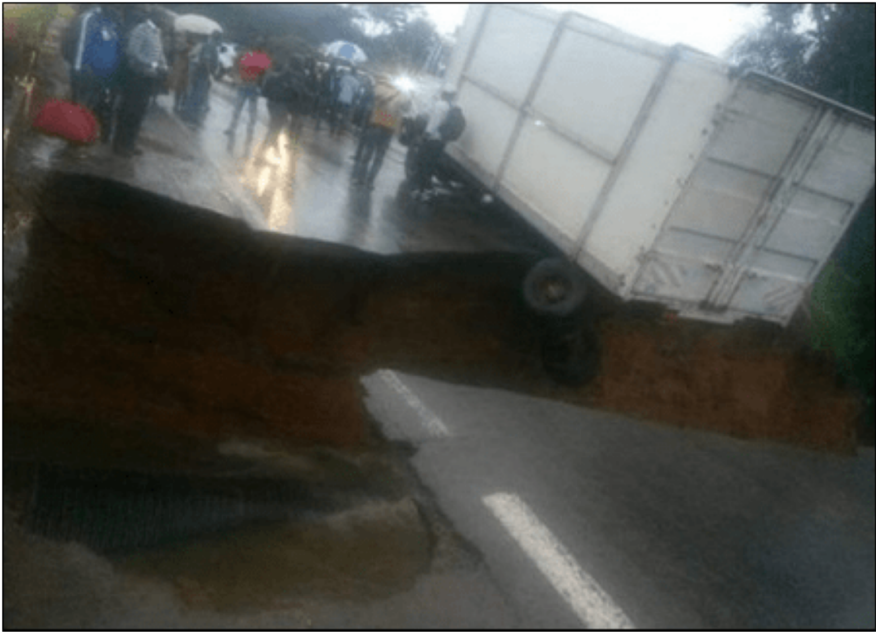
Figure 2. The rupture of the Manyai culvert, which forced people to head for the passenger station to get to Douala. Source: Copyright LCCLC/Facebook.com.
