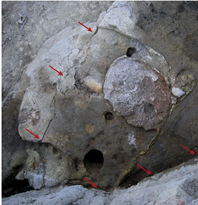
Figure 11 Photograph showing cracking around H03/13
