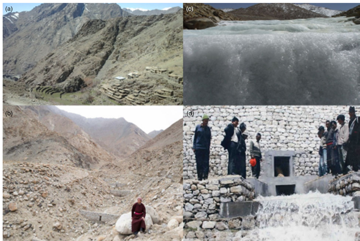
Fig. 1. (a) Site identification for construction and community area benefitted by artificial glacier. (b) Stone embankments constructed to build water reservoirs. (c) Freezing process of water over layerings. (d) Water discharge for early sowing.
