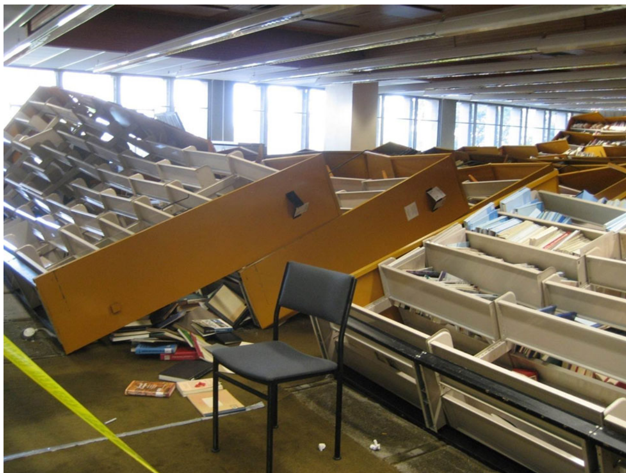
Figures 2: Collapsed shelves in the Central Library. Photo: University of Canterbury
