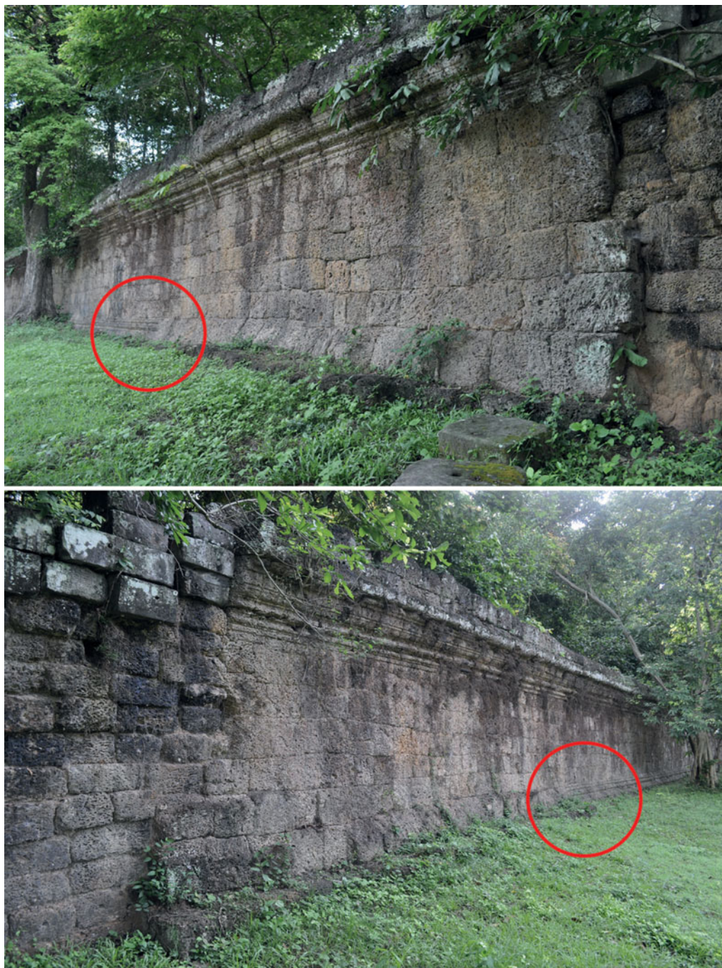
Figure 6. Gateway gap in the south wall, west side, facing west (top) and east (bottom); note the unfinished surfaces along the bottom edge of the wall adjacent to the gateway gap and the finer detailed blocks located farther away.
