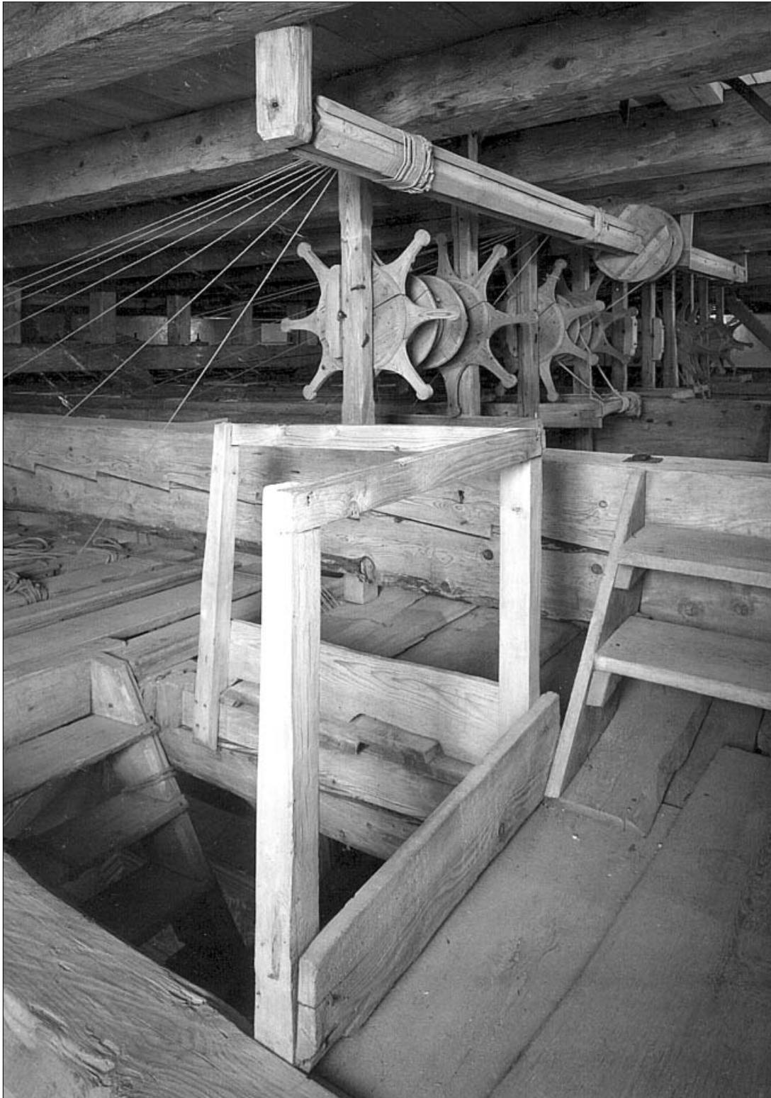
Opposite page: view from the gridiron of the Castle Theatre (photo: B. Marschall). Above: winch in the gridiron (photo: V. Skrabánek).
