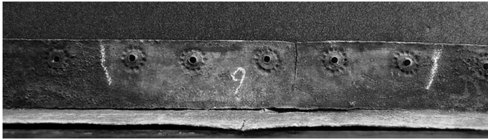
Fig. 4 Corrosion shadow on the underside of the edging-strip in position R6 showing position of a band, probably BM 124662
