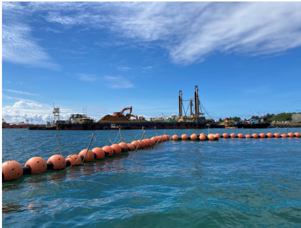
At the construction site in Ōura Bay, © Palz 2021. Every weekday ships and trucks bring soil for landfill.
