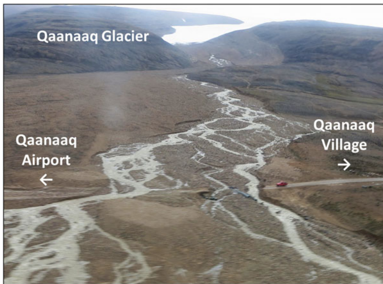
Fig. 1. Aerial photograph of the destruction of the road linking the settlement of Qaanaaq to Qaanaaq Airport by the outlet stream from Qaanaaq Glacier. (Photograph was taken on 3 August 2016, from a helicopter).
