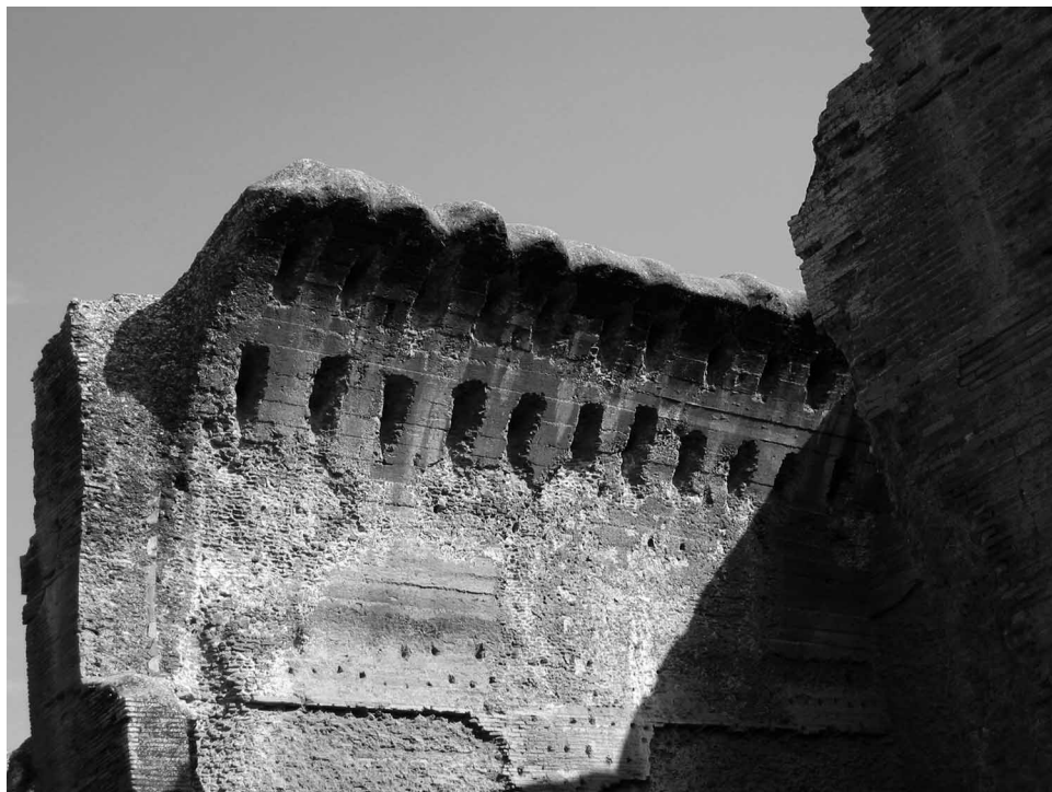
Figure 11. The tepidarium in the Large Baths in Hadrian's Villa, Tivoli. Remains of the barrel vault, laid on formwork boards supported by a centering structure. The room has a square plan, measuring 11.48 \times 11.48 m; the vault springs at over 7.2 m from the floor level. A large fragment of collapsed vaulting lies in the room. Clearly evident is the damage caused by the removal of the metal bars supporting the grid for the hanging ceilings. In this case, the first 45 cm from the spring of the vault has been chiseled away to extend the vertical wall upward for approximately 45 cm so that tubuli could be attached, as shown by the holes left by the T nails.
