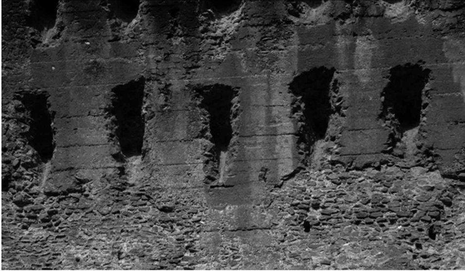
Figure 12. Tepidarium vault, detail, in the Large Baths in Hadrian's Villa. Evident in the concrete of the vault are the imprints left by the bars, which are nearly vertical. The holes are cut about 1 m deep.
