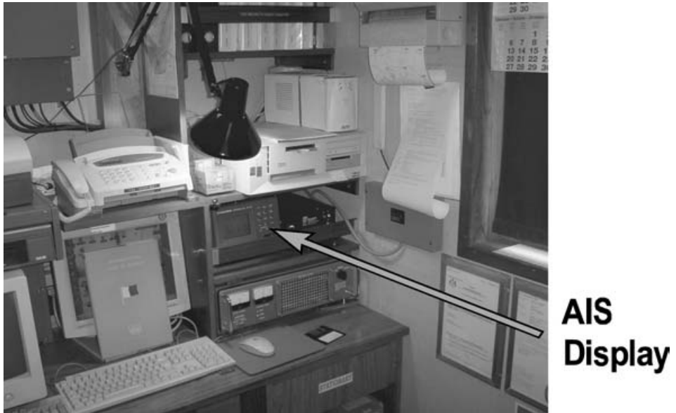
Figure 4. Poorly located AIS unit.
