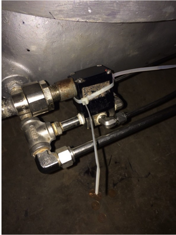
Photo from an inside source reveals the solenoid bypass which led to the June 2016 leak
