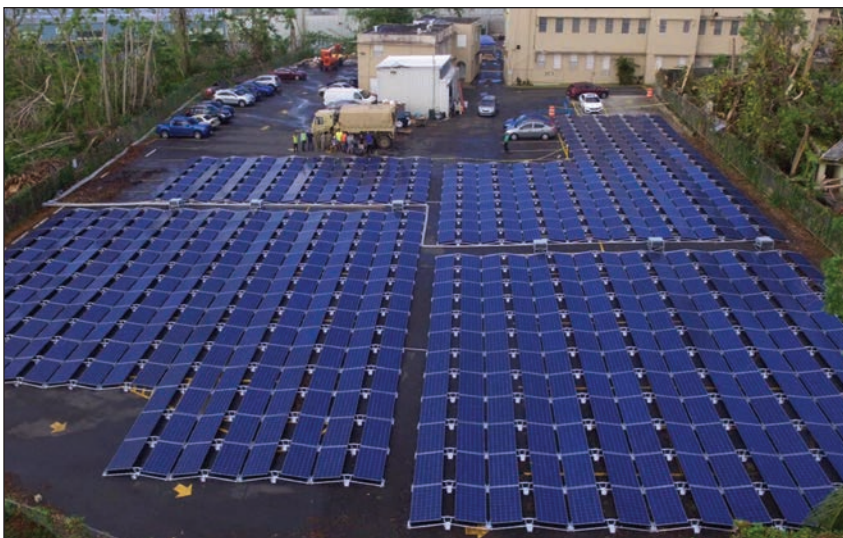
Tesla's solar power system generates electricity for Hospital del Niño in San Juan that serves about 3000 children across the island of Puerto Rico. Before the system installation, the hospital was forced to run off generators and ration diesel fuel. Photo credit: Tesla, Inc.
