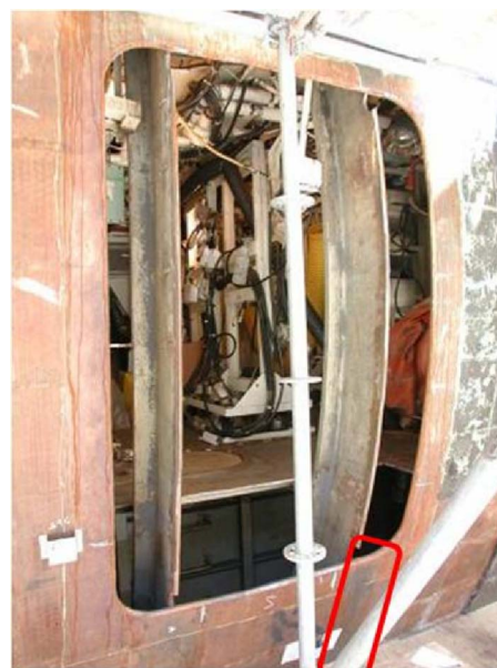
Figure 5. (Color online) Photograph showing the pressure hull of submarine B after removal of the affected plate. The location of the circumferential berthing weld is shown with a red box.
