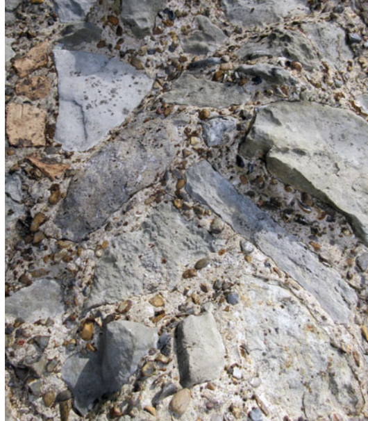
FIG. 8. Detail of the bonding mortar (a pebbly opus caementicium ) in a section of the Landward Wall by the Wardrobe Tower, Tower of London, made of 20-mm sized black round pebble flints bonded in a hard, chalky lime cement (image by K. Hayward).
