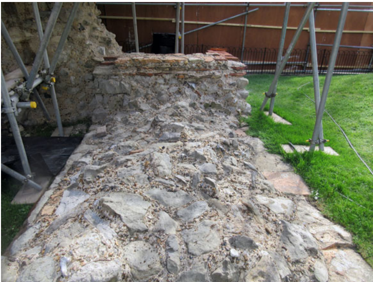
FIG. 7. Section of the Landward Wall by the Wardrobe Tower, Tower of London, showing a detailed view of the opus caementicium core with Kentish ragstone rubble pieces (photo by K. Hayward).
