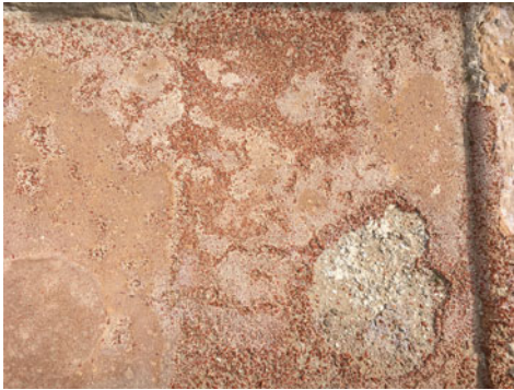
Figure 1. Roman opus signinum from a domestic cistern in Lucentum (Alicante, Spain). Note the remains of the smooth surface (left); smoothing closes the pores, thus improving impermeabilization. Here, the lining was applied on top of a base layer of sand-lime mortar.
