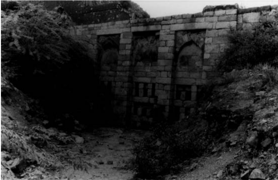
PLATE XXVI. Sluice gate near the ‘Ādilābād Gate seen in 1992 from the lake looking east towards the water outlets, before a modern retaining wall was built for the main road passing south (right) of the feature.
