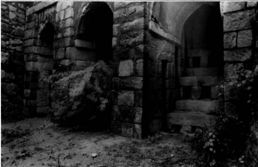
PLATE XXVII. Sluice gate, view from the east showing the water channel and the arches of the outlet housing the sluices. Three levels of openings for controlling the water can be seen.
