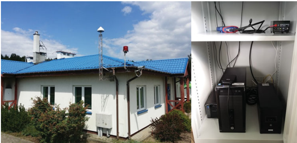
Figure 2. (Colour online) GNSS antenna and computer set with GNSS receiver installed in the building of the Aeroclub of Warmia and Mazury.
