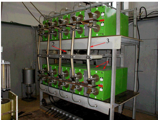
Fig. 8. (Color online) General view of the capacitor bank: 1 = capacitors, 2 = main switch, 3 = protective resistors.
