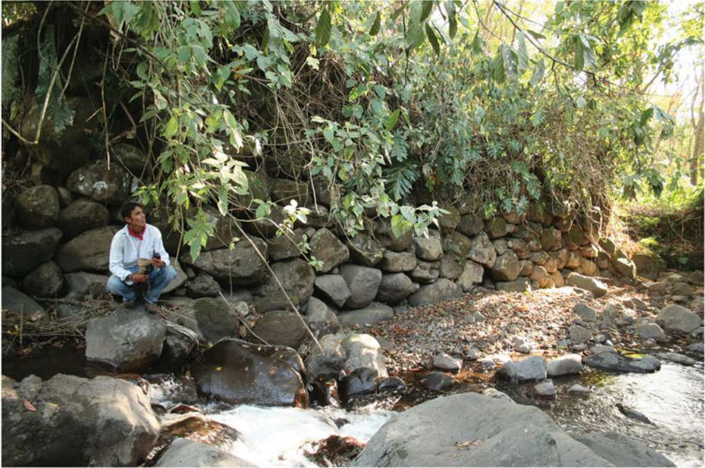
Figure 7. West abutment of the Ichanhuehue bridge during the dry season in late 2010 (photograph by Oswaldo Chinchilla Mazariegos).
