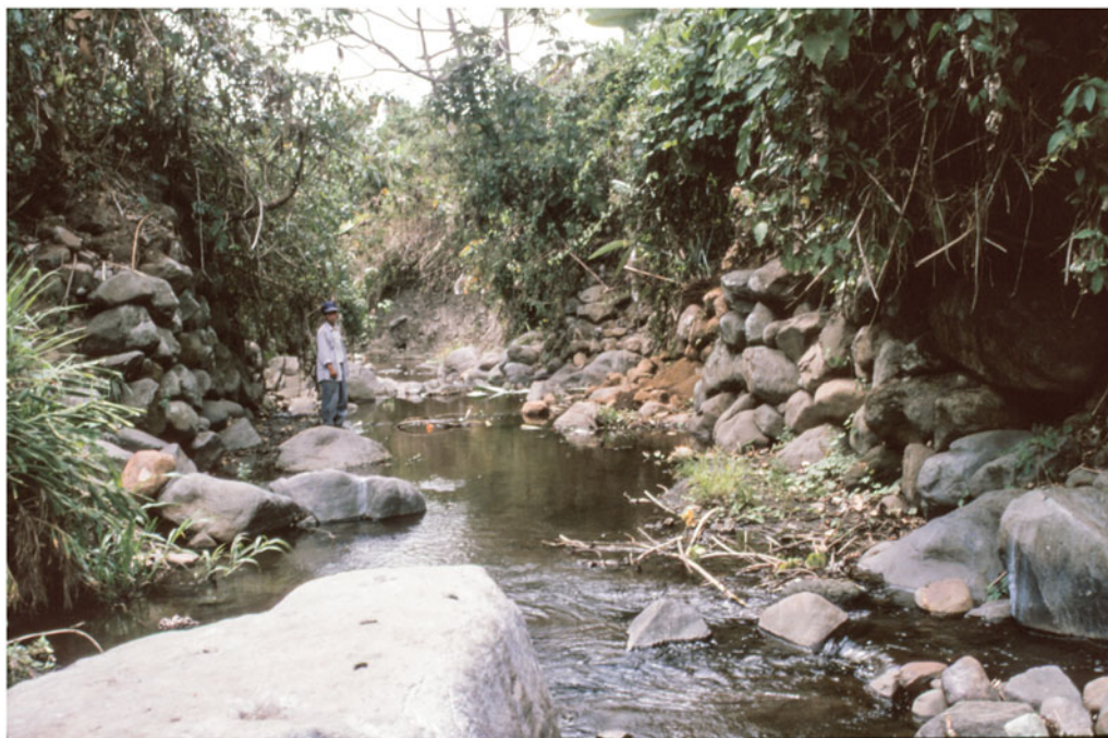
Figure 3. Abutments of the El Baúl bridge. View to the south, taken during the dry season in 1997 (photograph by Oswaldo Chinchilla Mazariegos).
