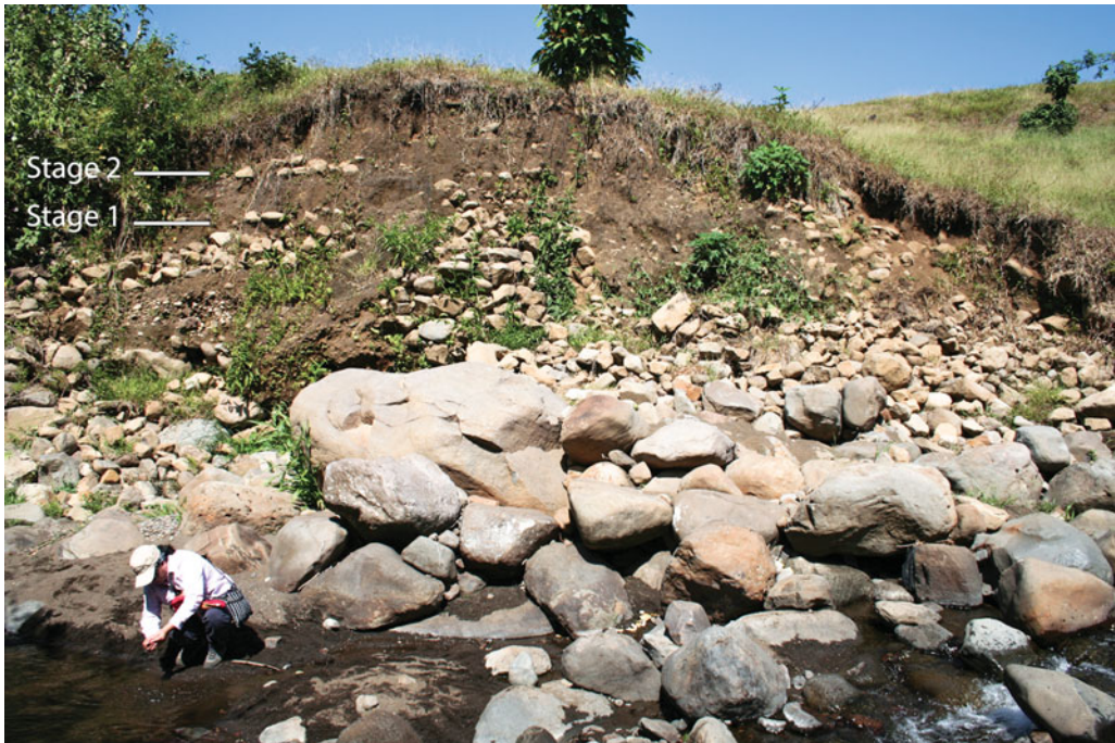
Figure 6. The northern side of the El Baúl bridge in late 2010, after Tropical Storm Agatha washed away the abutment, revealing the artificial fill that was deposited to raise the approach to the bridge. Note the superimposed pavements of construction stages 1 and 2 of the causeway. Blocks from the dislodged cyclopean wall are still visible in the foreground (photograph by Oswaldo Chinchilla Mazariegos).
