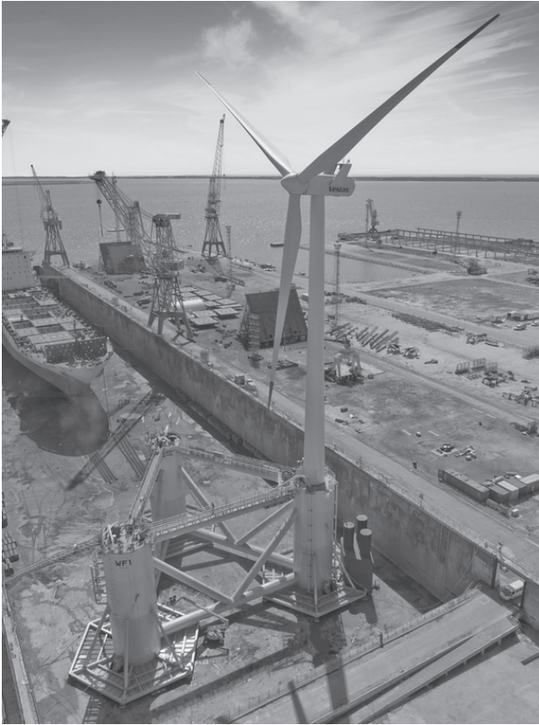
Figure 1.6 The floating wind turbine Windfloat 1 during construction in Portugal. Note the heave plates whose function is to increase the vertical added mass, shifting the heave and pitch natural periods out of the wave period range. Additional benefit comes from decreased wave excitation loads and increased viscous damping (courtesy Principle Power, Inc.).
