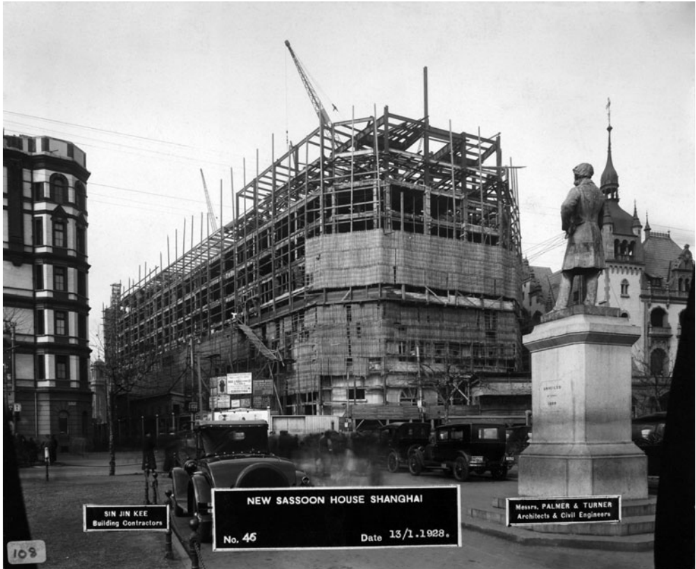
Illustration 5. Sassoon House (The Cathay Hotel) under construction, Shanghai, January 1928. Reproduced with the permission of Teesside Archives, reference BS 1829.
