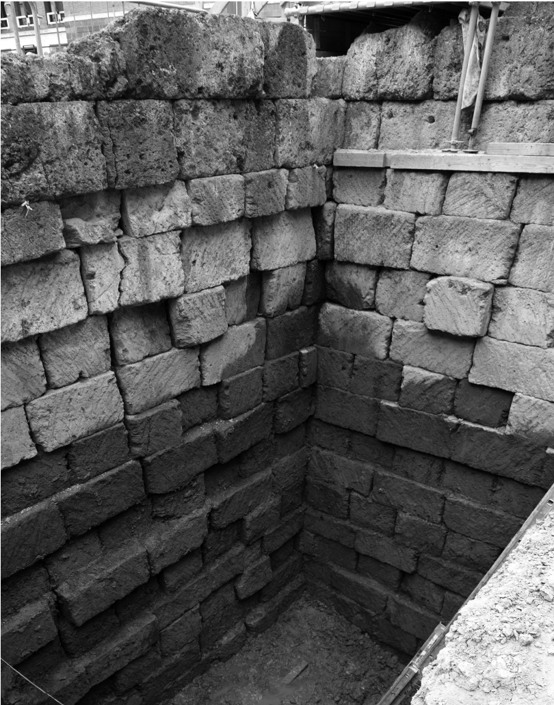
Fig. 9. Tufo del Palatino foundations of the W cella in Sounding A7, looking southwest (D. Diffendale).
