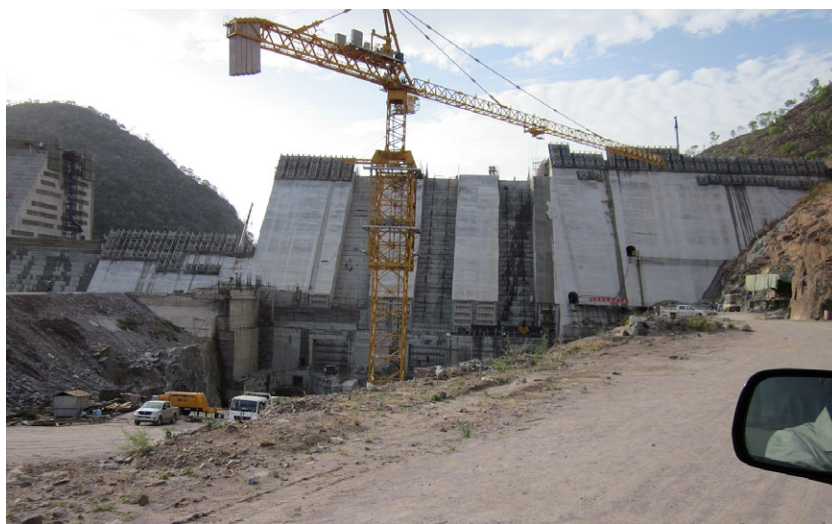
Figure 2. The Bui Dam under construction, February 27, 2011. The steps in the three channels for the dam's penstocks (behind the crane) correspond to RCC layers. Photo by author.
