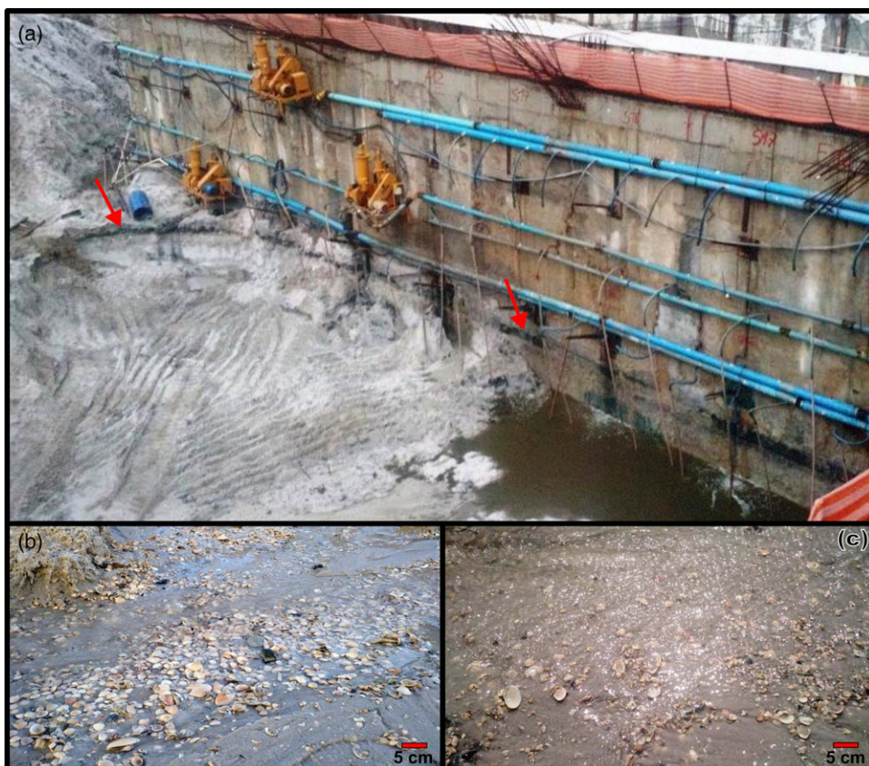
Figure 4 (a) Quartzose sand intercalated by a dark muddy layer (indicated by red arrows) that left traces in place on the surface of the retaining wall, at 6.3 m depth underground. (b) and (c) Shells found on the excavation site between -10 and -9 m. Photographs kindly provided by engineer Roberto Almeida.
