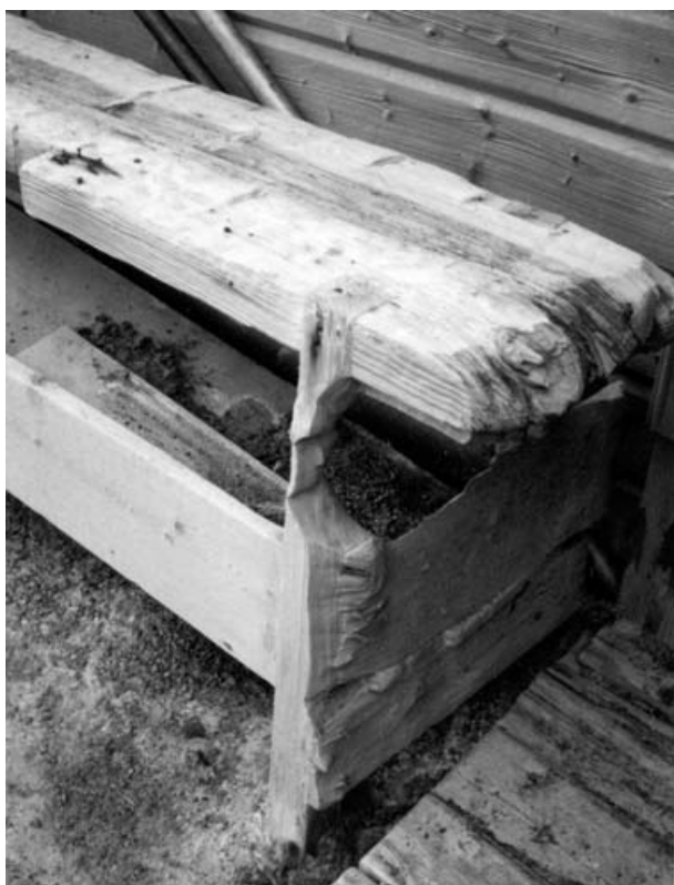
Fig. 6. Severely weathered end carpenter's work bench. January 1990.
