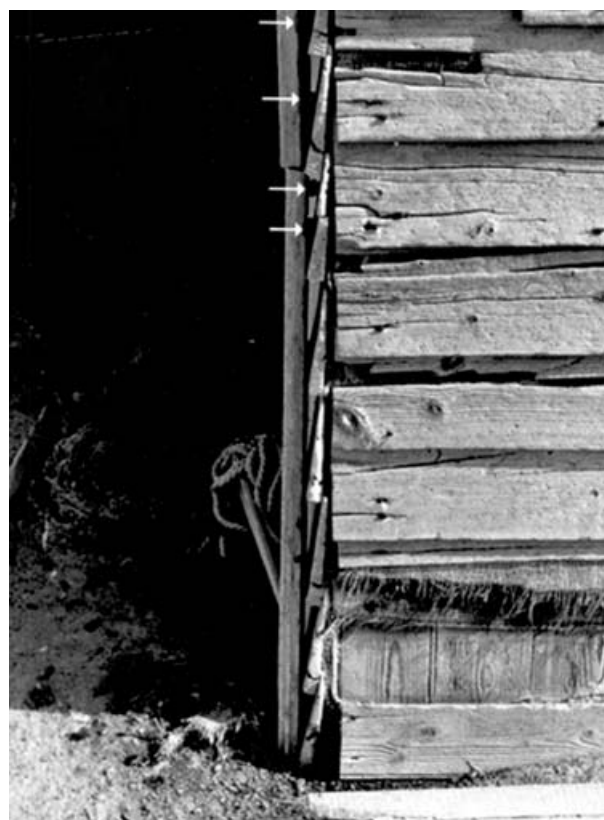
Fig. 8. Pebbles embedded between boards of porch wall 1911 hut. January 1990.
