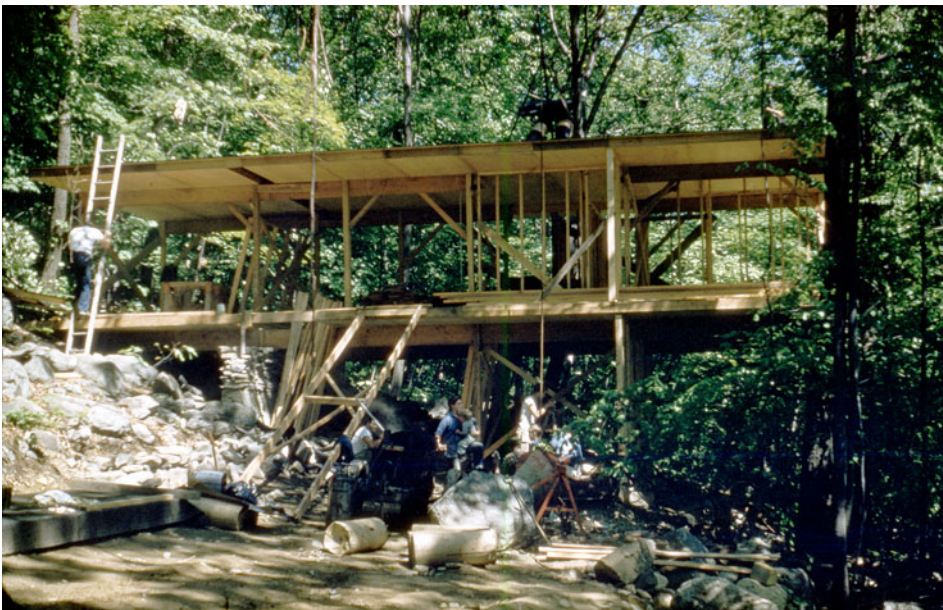
Figure 10. (Color online) Construction site: “Williams-Cage” house, 1955. Photograph by Richard Hora. Courtesy of Mies Hora.
