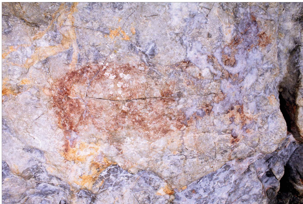
Figure 2. Panel 2, graphic unit 3, which has been affected by calcite formations and humidity (figure by the authors).
