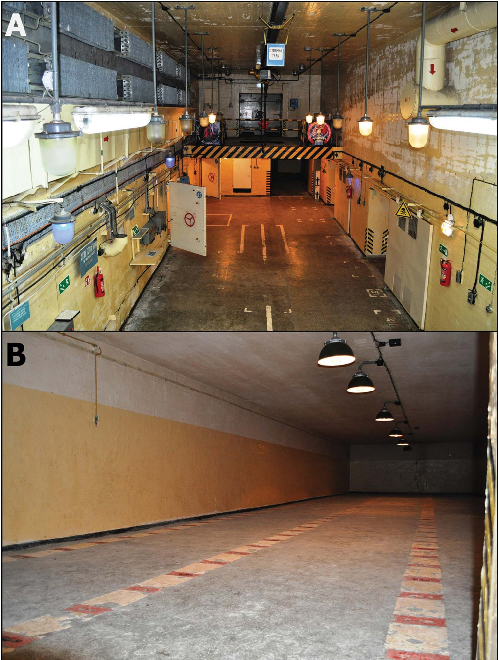
Figure 4. Interior of the Monolit bunker in Podborsko, with its original furnishings: A) main chamber with crane, loading ramp, and cooling and ventilation systems; B) one of four rooms used for storing nuclear warheads (photographs by G. Kiarszys).
