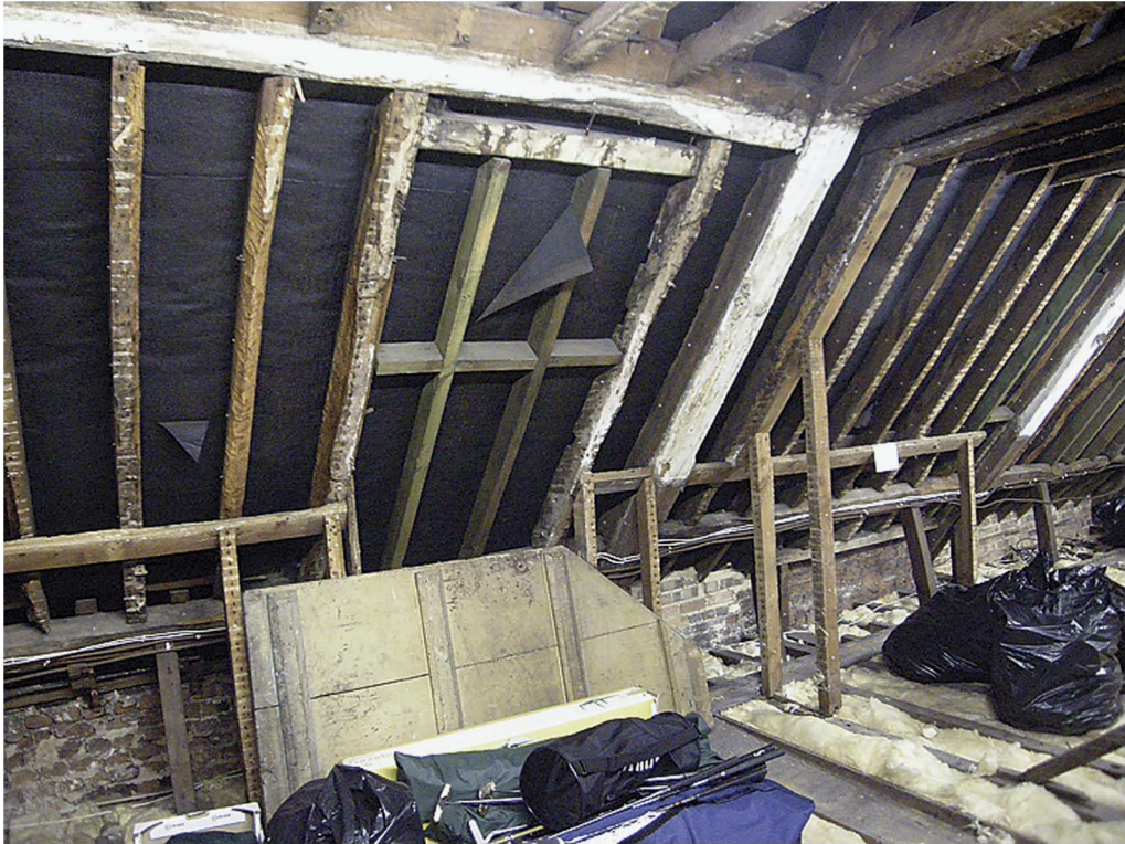
Fig 11. Moor Park: blocked dormer window position on the courtyard side of the east range. Photograph: Sally Jeffery
