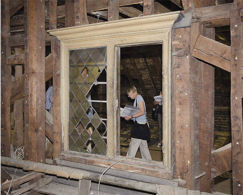
Fig 10. Moor Park: external face of central casement window in garret, relocated within framing of Thornhill's structural partition. Photograph: David Wrightson
