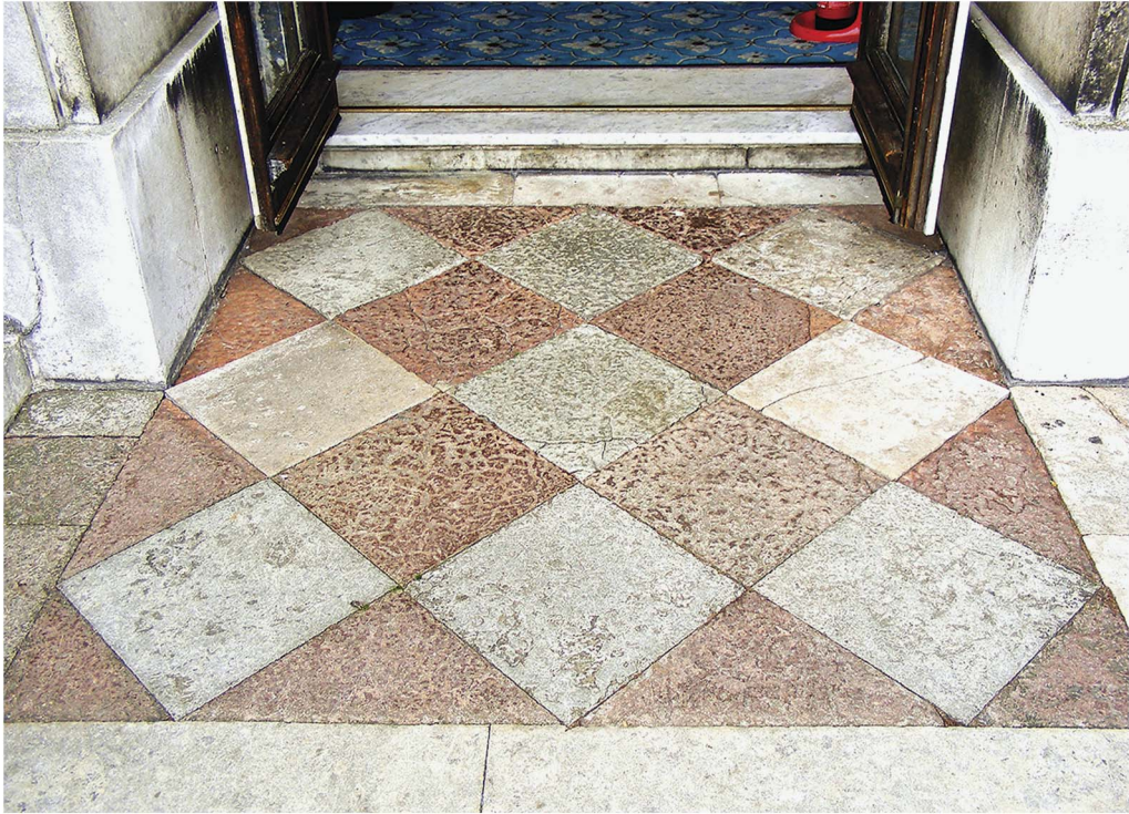
Fig 6. Moor Park: paving laid 'Arrace Way' outside the central door on the east.
