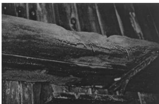
Fig. 7. Chemical spill inside the Cape Evans hut causing a deterioration of the wood. High concentrations of chromium and lead are associated with this caustic chemical spill.
