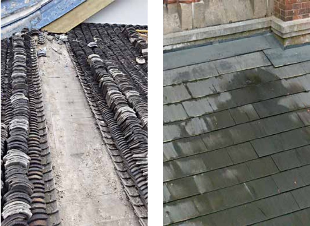
Fig. 8. Comparison between Chinese blue tile (left) and English slate (right) roofing: Denghui Building, Fudan Middle School, Shanghai, 1904, photograph of 2019 by Qin Yue; and Trinity Church, Shanghai, George Gilbert Scott, 1869, photograph of 2023 by Hongbin Zheng
