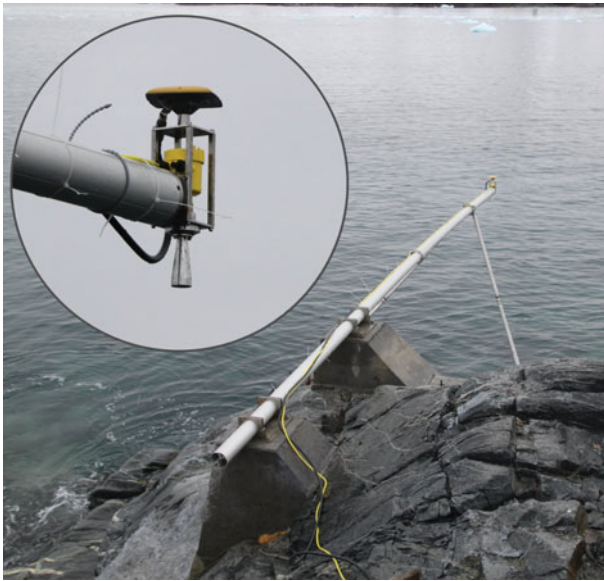
Fig. 7. (Colour online) Installation of the radar gauge system. Inset shows detail with GNSS antenna on top and radar waveguide below.
