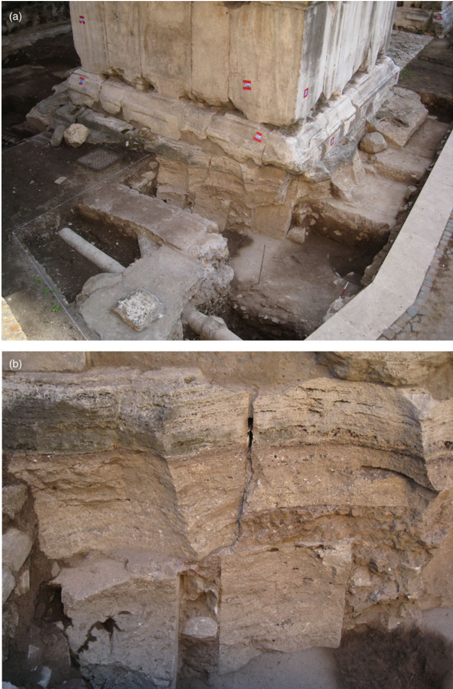
FIG. 2. Archaeological excavations in the foundations of the north-west pillar and detail of the construction technique, showing mortar in the joints between the blocks.
