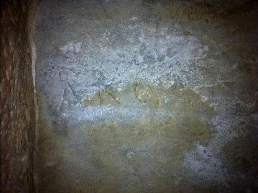
FIG. 13. New inscription B-5 documented in our architectural analysis inside the arch, north-west pillar.
