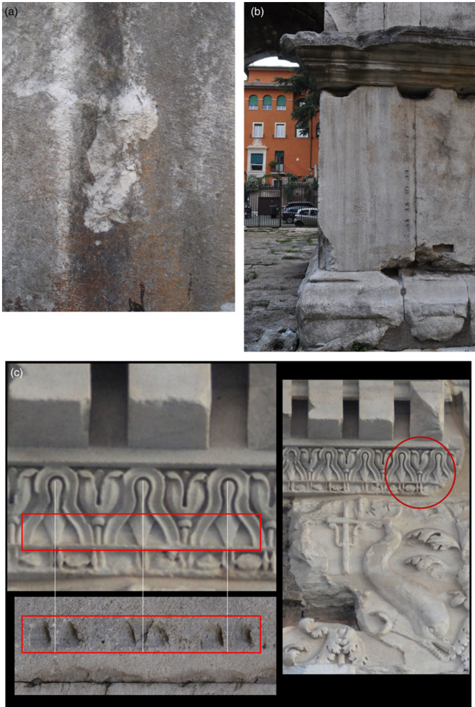
FIG. 6. Decorative elements from sections that were re-used in the construction of the arch. (a) Detail of the winged image of Victory eliminated as the architectural element was fitted in place; (b) architectural element with Bügelkymation eliminated for re-use as a block in the north-west pillar; (c) detail of the Bügelkymation in the cornice of the Hadrianic Basilica Neptuni.
