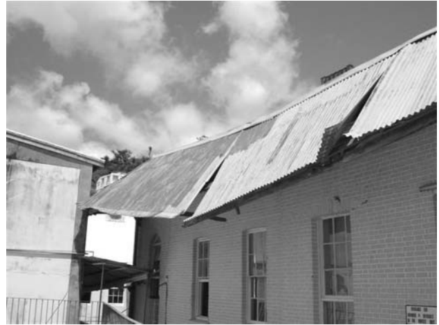
View from Sir Archibald Law Library showing part of roof over courtyard following devastating hurricanes.
