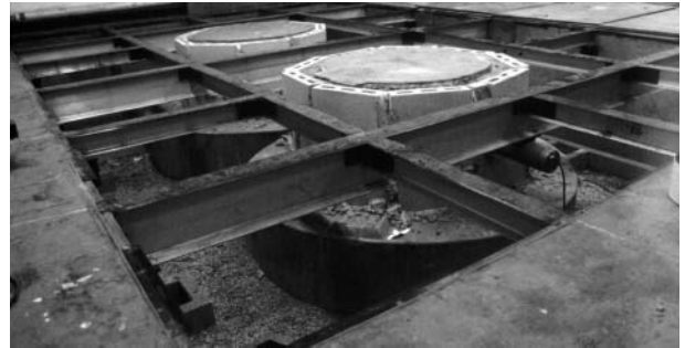
Figure 1. Exposed girder system of The Live Room with two vibration isolation pads, floor plates removed.
