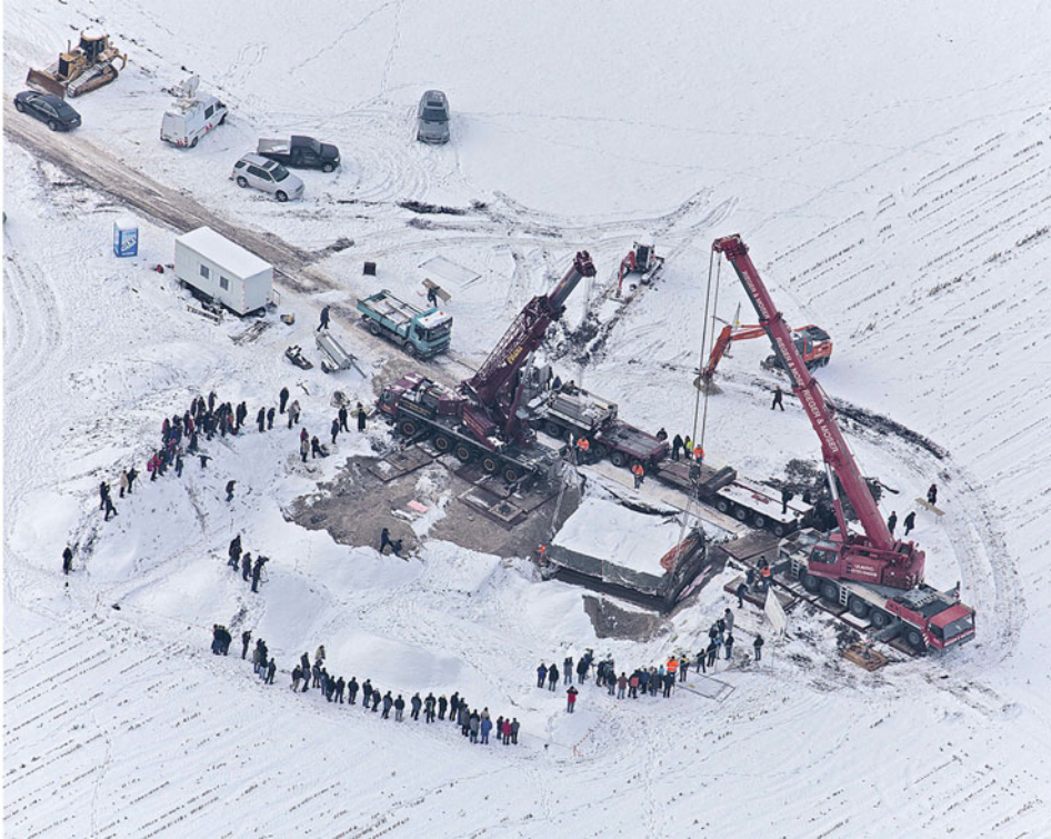
Figure 2. An aerial view taken on 28 December 2010 of the 80-tonne block being raised.
